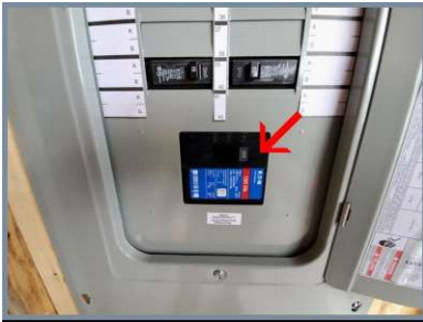
200 amp main circuit breaker.
