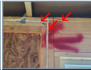
Wall not connected at front wall loft.
