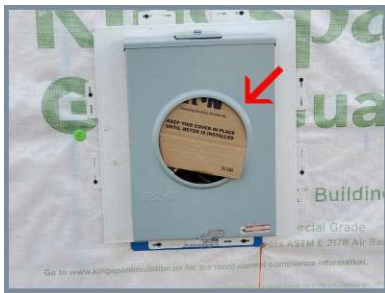
Underground electrical service.
