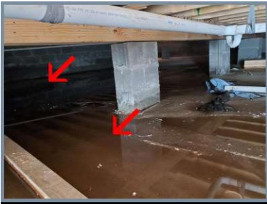
Standing water in crawlspace.
