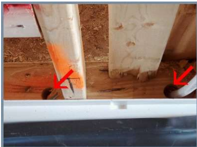
Missing fire stopping master bath shower.
