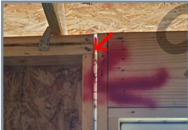
Separated wall in 2nd floor loft.
