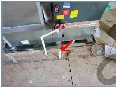
Incomplete over flow drain.
