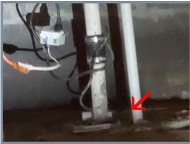
Sump pump in crawlspace.
