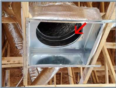
Air return vent.
