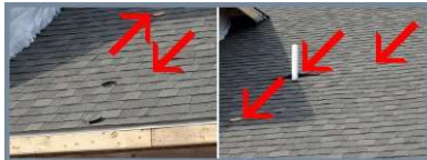
Open Roof penetrations.
