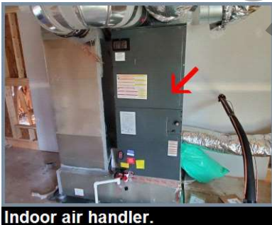
Indoor air handler.
