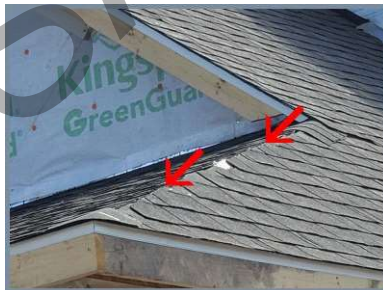
Incomplete roof material.
