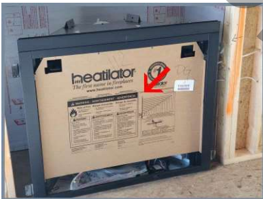
Gas fire place.
