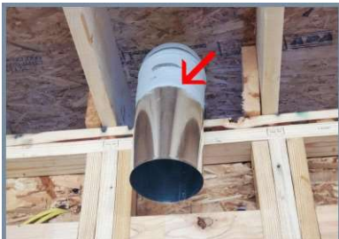
Kitchen vent ductwork.
