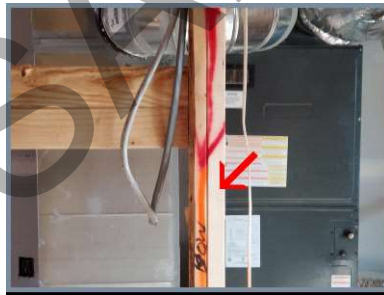
Bowed wall stud at second floor bedroom.
