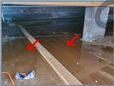
Water at crawlspace floor.
