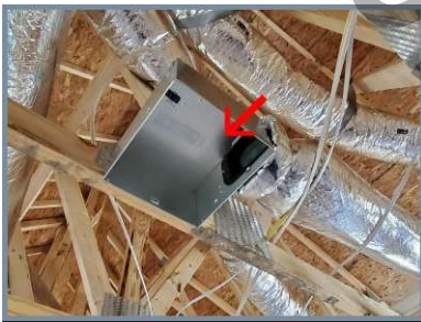
Bath vent and ductwork.
