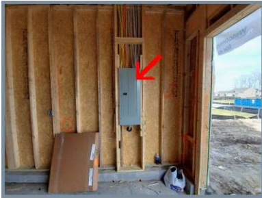
Main electrical panel in garage.
